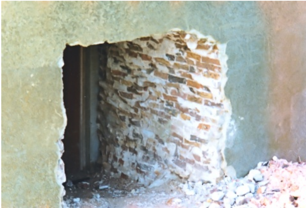
New entrance being made in the seaward side of Martello Tower No.23 in 1989
